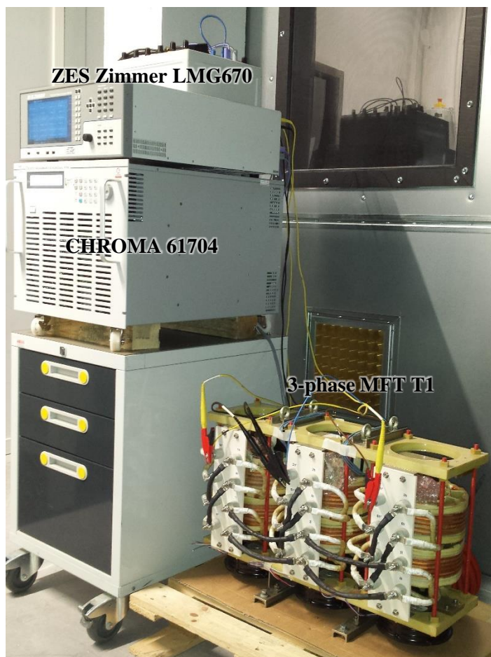
Fig. A14. MFT T1 no load test with a variable frequency 3-phase sinusoidal power supply
