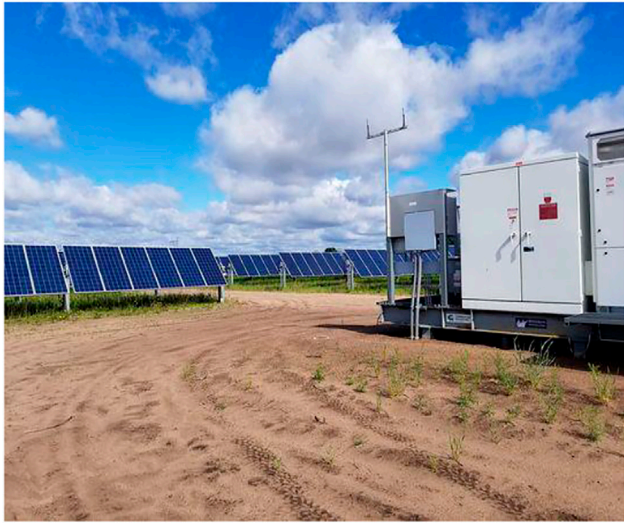
FIGURE 1 | Photovoltaic system (Flickr).
