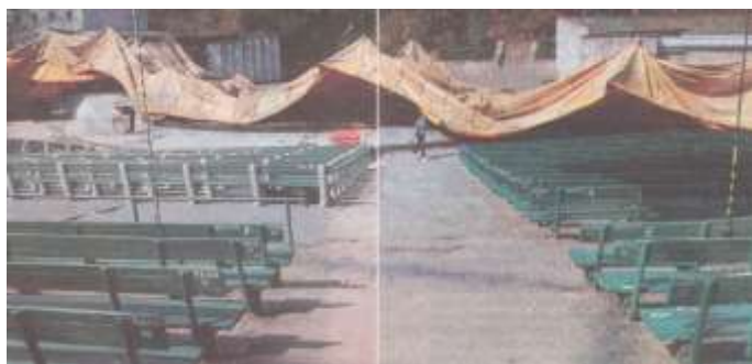
Figure 1. Putting down the roofing structure of the Forest Opera in Sopot (Poland) before winter season (Dziennik Bałtycki 2007).
