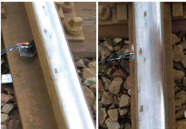
Fig. 3. Defect 221 – damage of the running surface on railway line no. 213 Reda – Hel [authors' own work]
