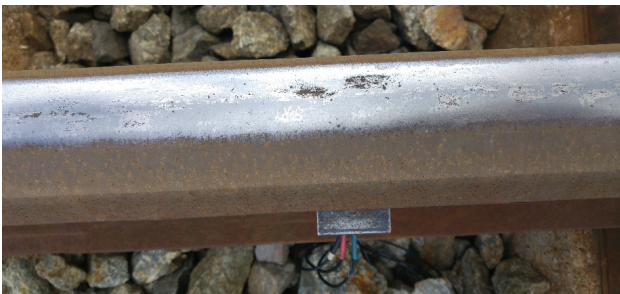
Fig. 2. Spalling defect on railway line no. 213 Reda – Hel [authors' own work]
