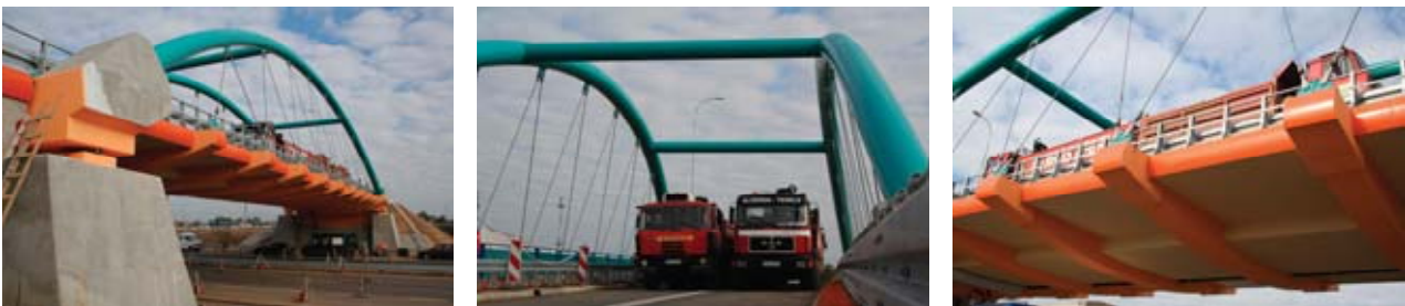
Fig. 11. Construction of the arch span of the viaduct in Nowy Dwór Gdański
