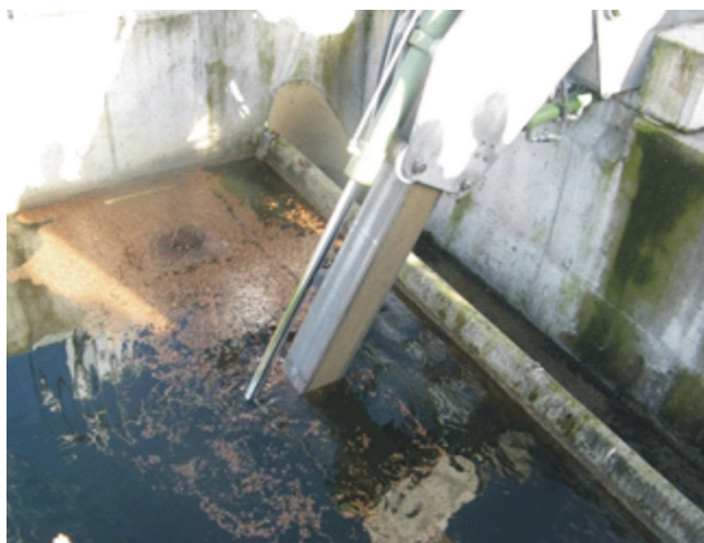
Figure 1. Purification of water from “thick” pollution at an SHP (photography: B. Igliński).
