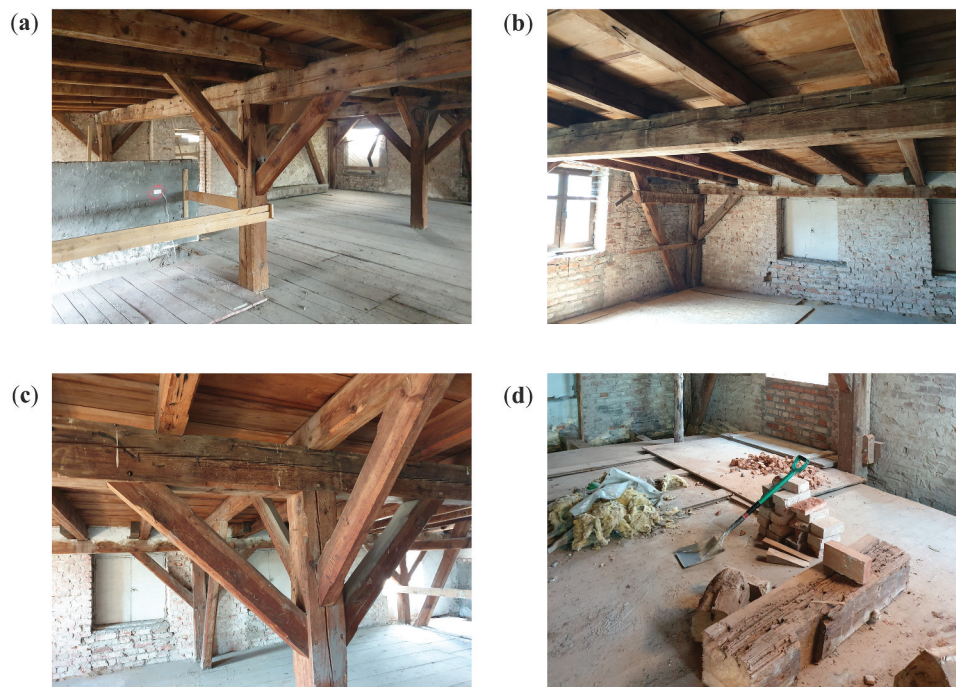
Figure 4. Photographs of the roof framework from the monastery of congregation of the sisters of St. Catherine in Orneta (Poland) before starting construction work (a-c) and when the works are carried out (d).
