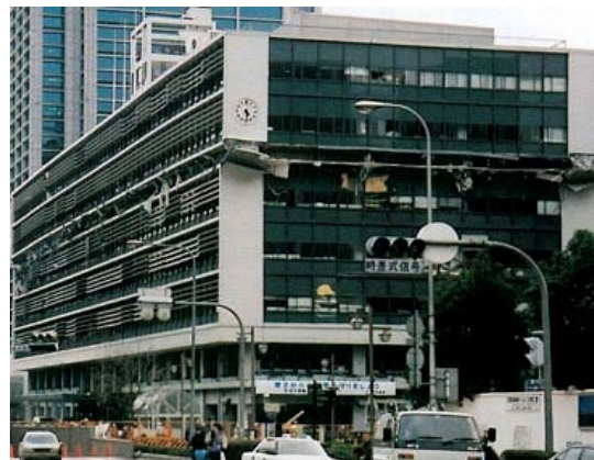
Fig. 1: Soft-storey failure of the intermediate storey of building (Kobe 1995)
