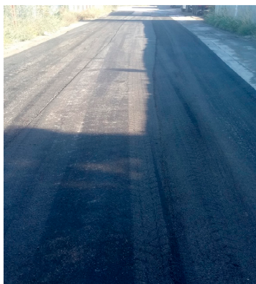
Figure 8. First short test section at the asphalt plant (MTM1) constructed during technological trials described in Section 3.6—September 2018.
