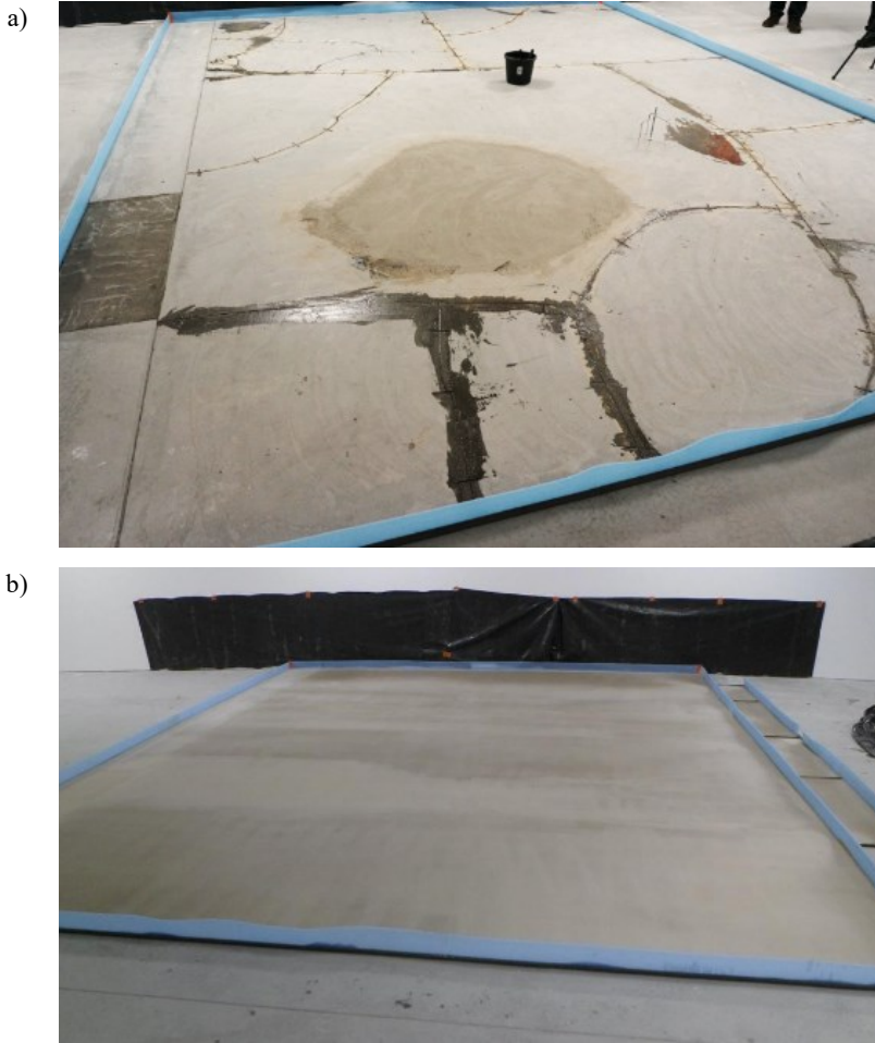
Fig. 13. Repair method: a) view after stitching and injection of the cracks, b) finished top layer.
