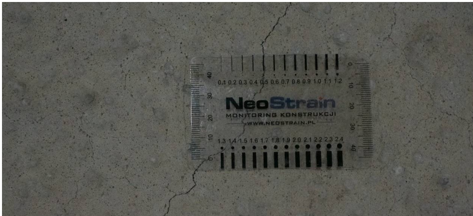
Fig. 10. Measurement of the cracks in sample no. 4.
