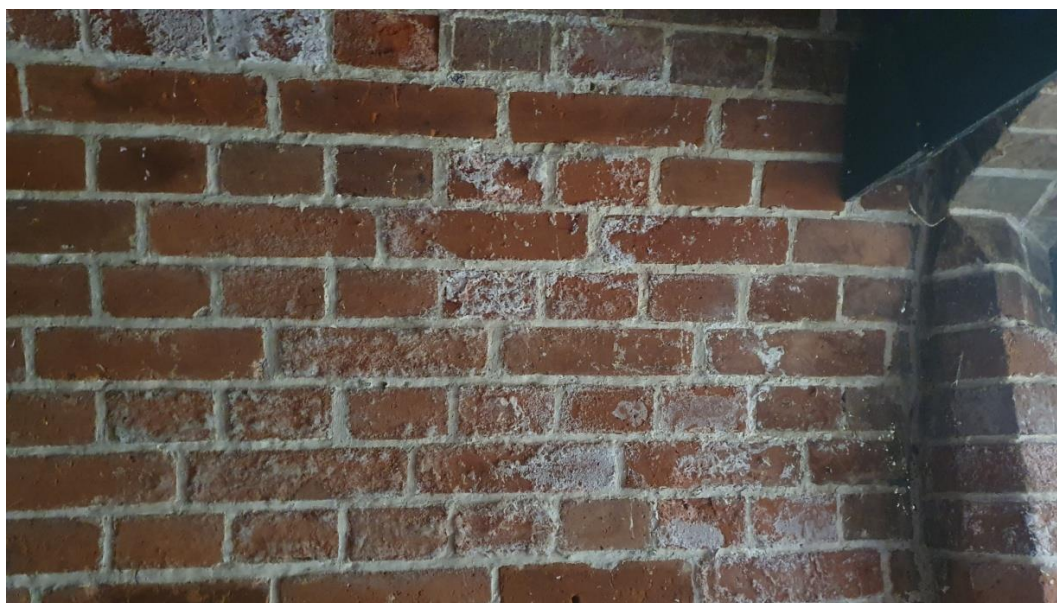
Fig. 4. Development of biological corrosion on the interior surface of the exterior solid ceramic brick masonry, visible cement mortar tight joint improperly executed in the past period during renovation work (photo: Maciej Niedostatkiwicz)
