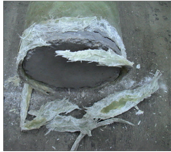
Fig. 2. Destruction (debonding) of a pipe made of glass fibre reinforced composite
