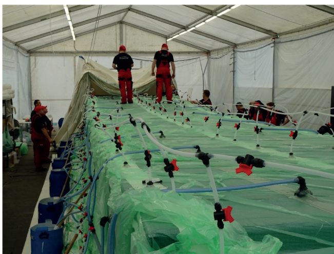
Fig. 2. Preparation to infusion of a large-size object - footbridge span of Fobridge grant
