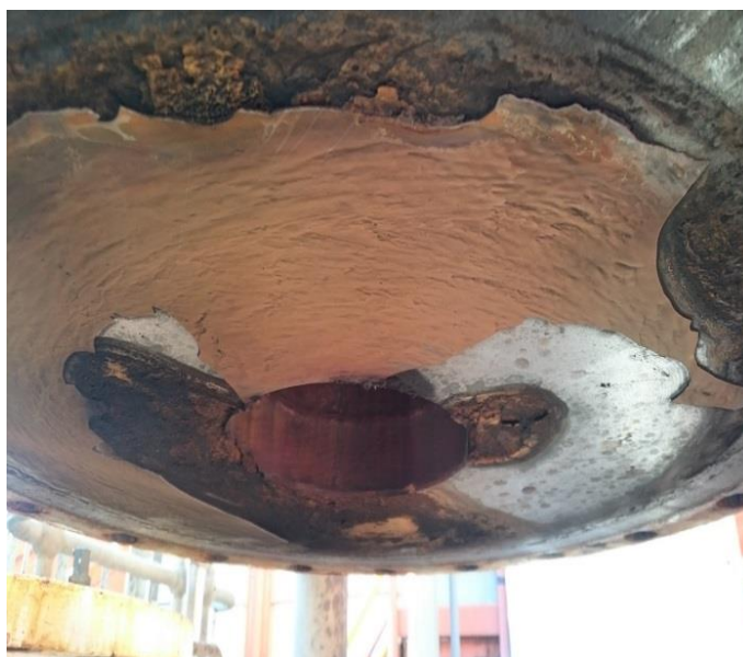
Figure 2. Surface of the inner parts of the dual media filter.
