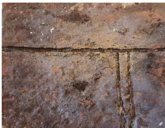
Fig. 2. DN 800 water pipeline – corroded section of the longitudinal seam and butt circumferential weld above
