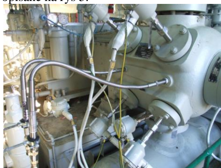
Fig. 6. Pressure sensors mounted in the compressor
