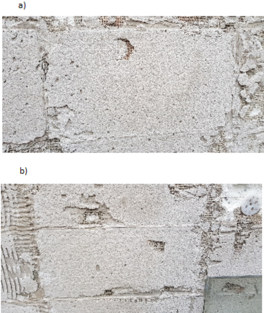
Figure 3. Mechanism a), b) (method of detaching) the ceramic cladding of the building facade
