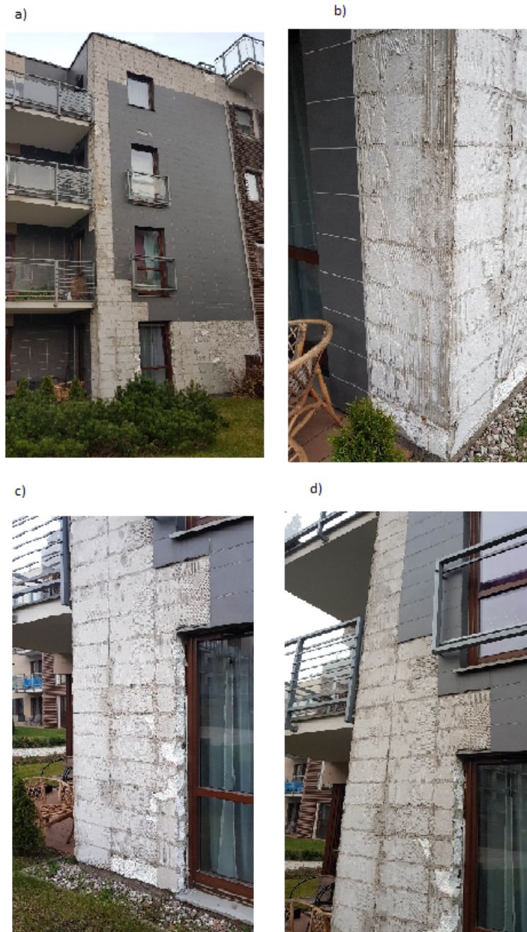
Figure 1. Damaged ceramic cladding a), b), c) and d) of the building facade
