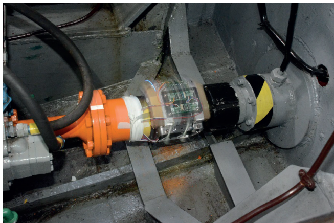
Fig.3. Torque and thrust measurement system rotating with the propeller shaft during the measurements
