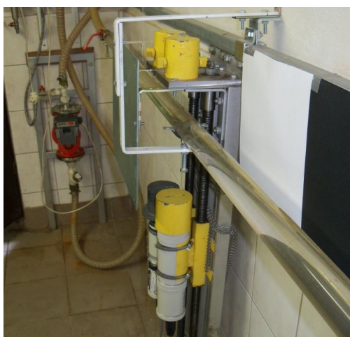
Fig. 2. A view of the measurement section of the installation.
