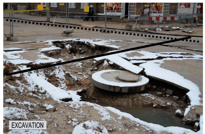
Figure 13. Close-up of the Gdańsk 2013 pipe failure area Dotted lines indicate road edges while solid line indicates the axis of the pipeline
