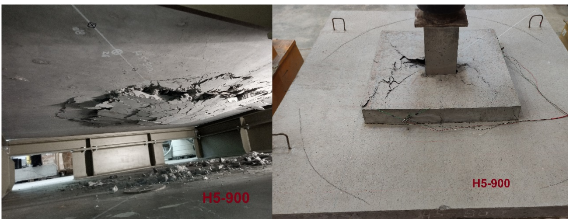
Fig. 11. Failure form of H5-900 element.
