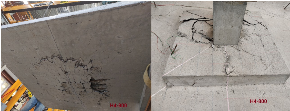
Fig. 10. Failure form of H4-800 element.
