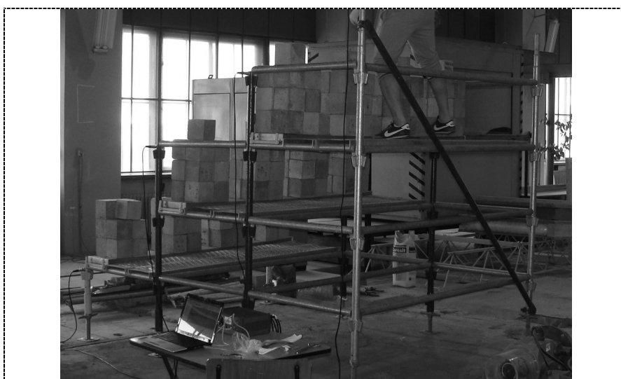
Figure 1. Steel temporary grandstand with typical diagonal stiffener.
