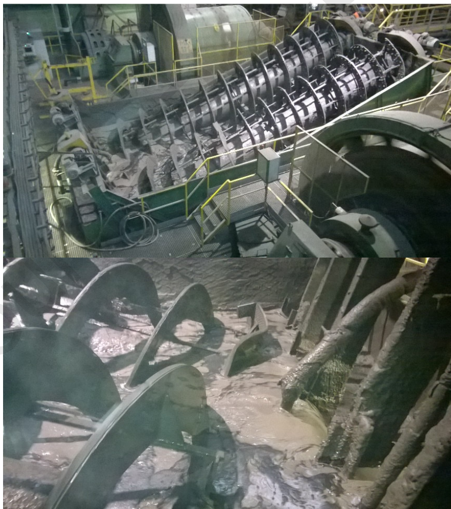
Photo 1÷2. Spiral classifier used in the process of copper ore classification.
