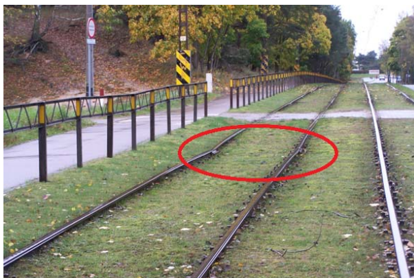
Fig. 3. Displacements of the sleepers in the track
