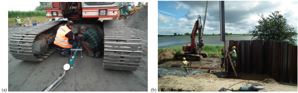
Fig. 5. Construction stages: (a) compaction verification – plate loading test (b) installation of sheet-pile wall
