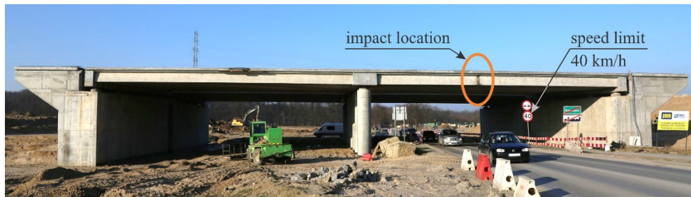
Fig. 1. Overall view of the bridge. The location of the impact is marked orange.
