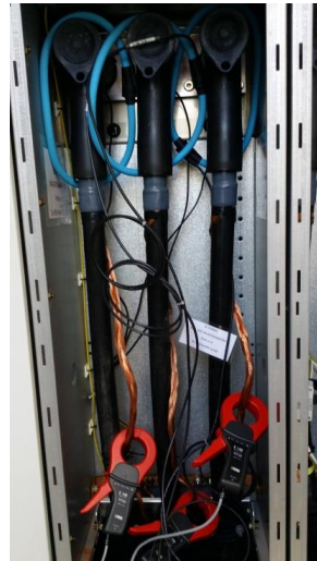
Figure 5. Measurement of currents flowing in cores and sheaths in Substation 2.
