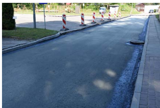
Figure 7. Unbound aggregate base course ready for laying the binder course made of AC 16W.
