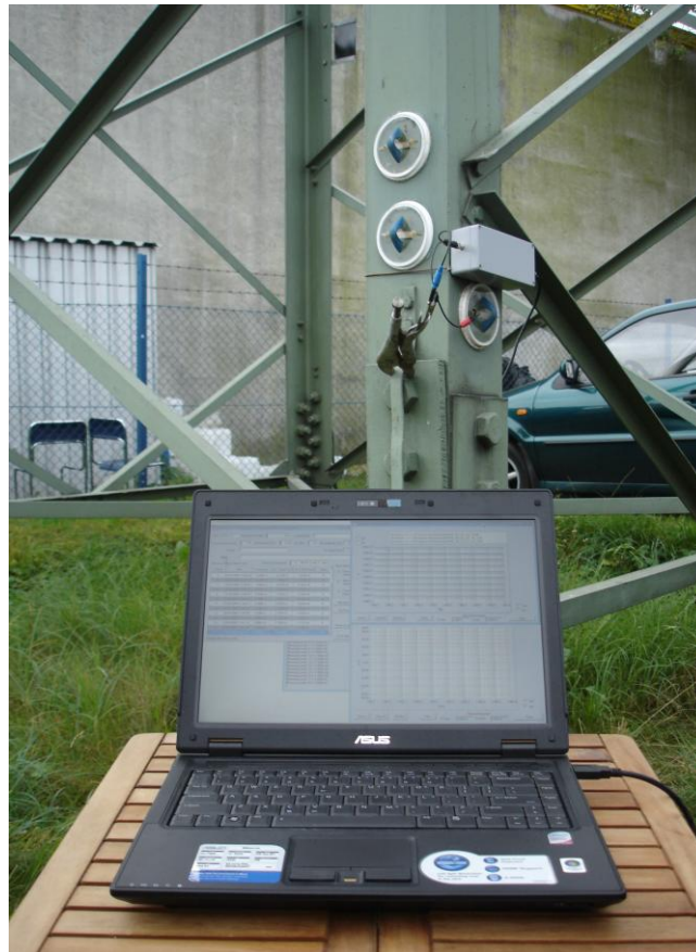
Fig. 8. Impedance measurements in the field of the anticorrosion coating on a high-voltage pylon, using the interface circuit powered and controlled by portable computer via USB
