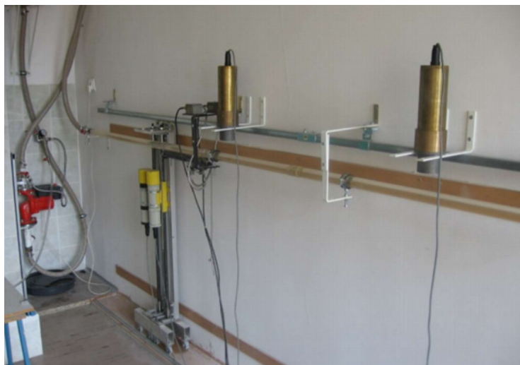
Figure 2. General view of the hydraulic installation.
