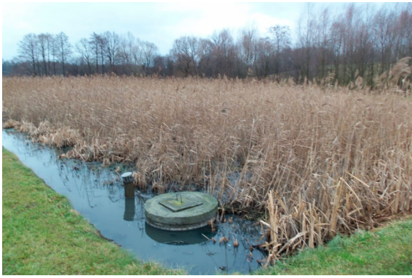
Figure 3. Clogging effect after 12 years of operation (winter season) at the TW in Inwałd, Poland.
