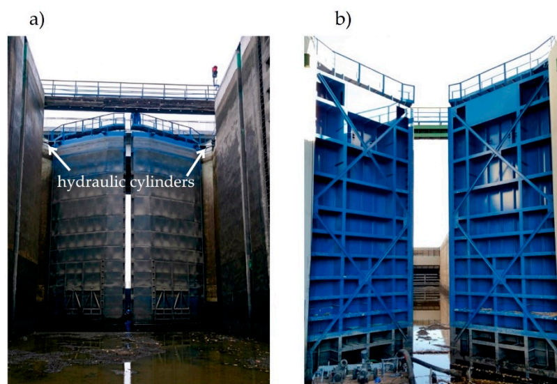
Figure 2. General view of the Wloclawek lock bottom miter gates. (a) From the side of the lock; (b) From the side of downstream.
