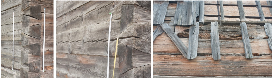
Figure 6. The church in Cewków: wall corner, longitudinal cracks in the wall, visible cavities in the wall.
