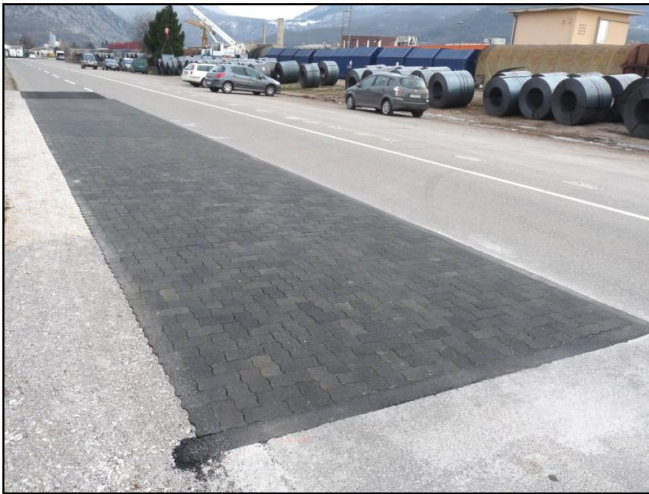
Figure 15: Just finished Slovenian full scale test track in Nova Gorica (Picture: D. Kokot)
