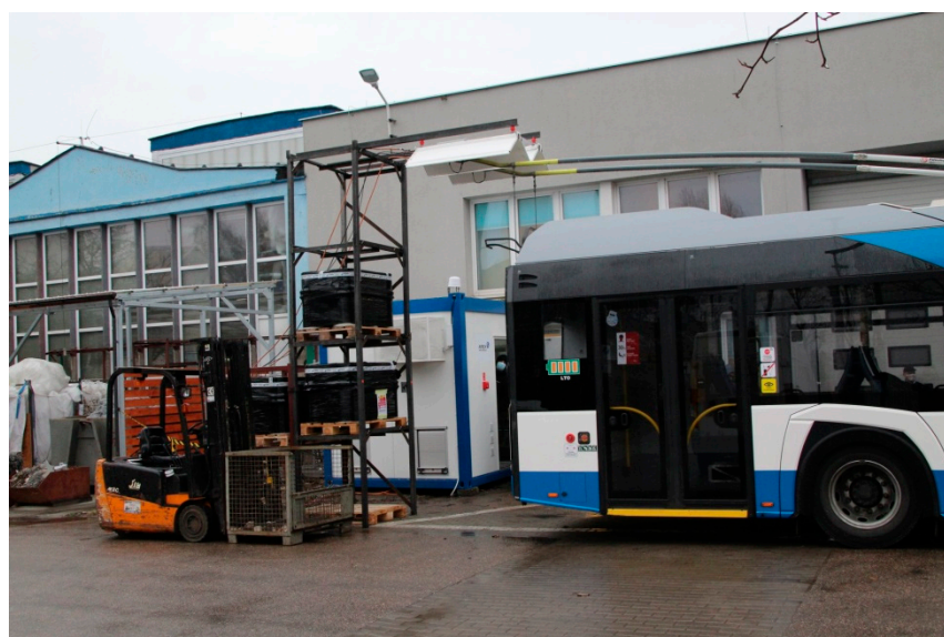
Figure 2. Technical tests of a prototype of a 150 kW fast charging station for trolleybuses in Gdynia (photo taken by M. Bartłomiejczyk).
