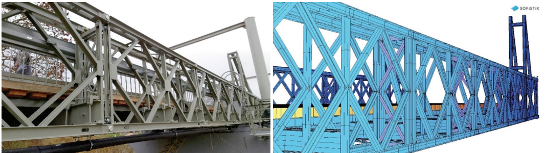
Figure 19. Bridge detail compared with the FEM model – side view of the bridge
