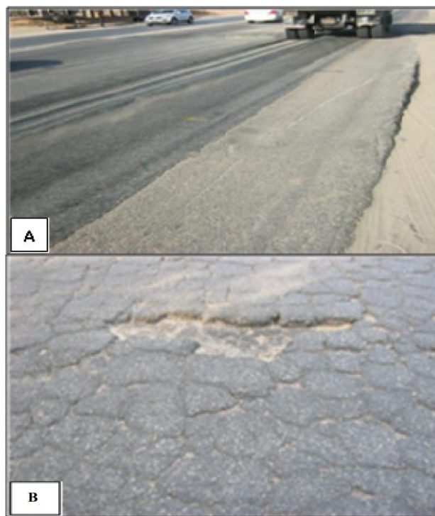
Fig. 2. (A) Rutting; (B) Fatigue cracking [16].
