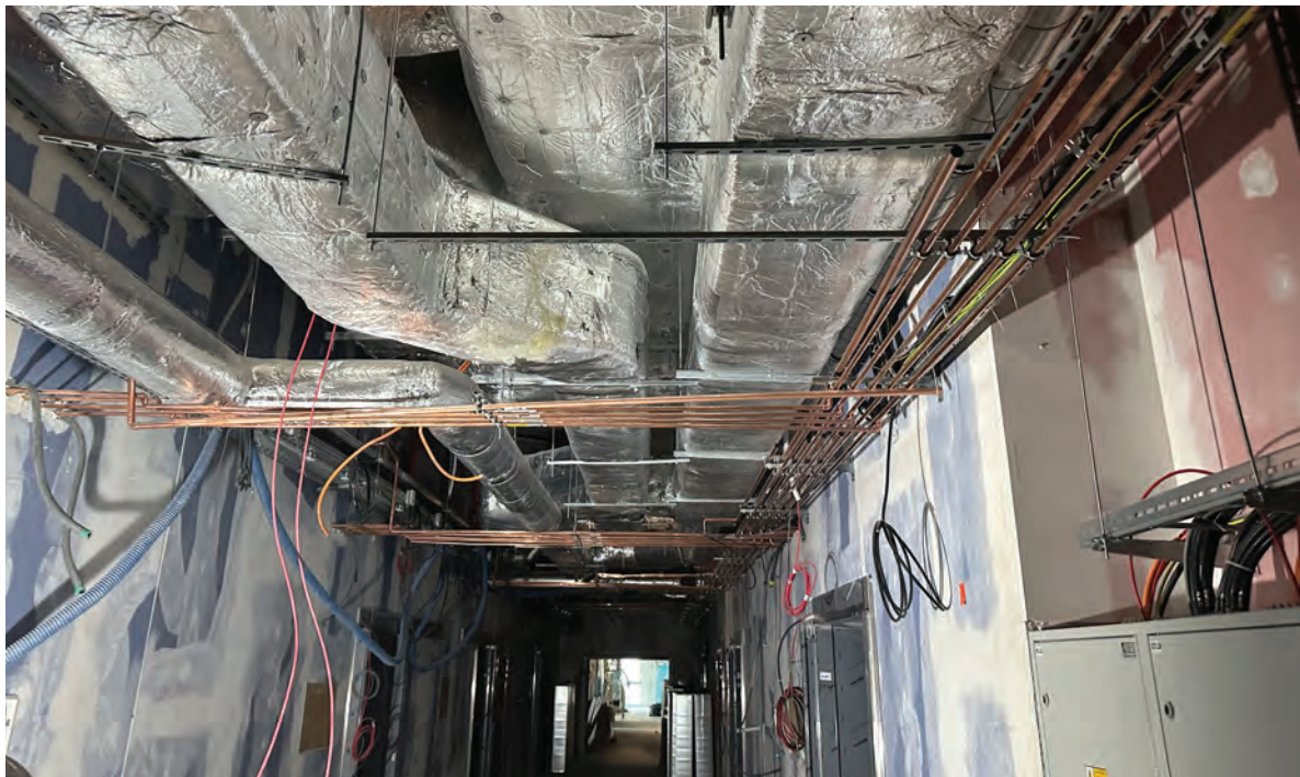
Photograph 3.1.1 A corridor (technical infrastructure in a modern hospital is an extended, complex structure that requires the HAI risk analysis); photographed by the Author, 2014
