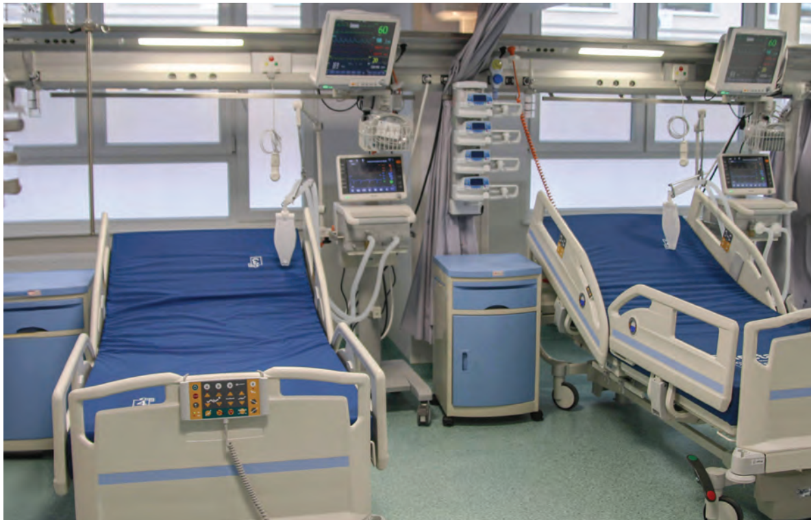
Photograph 6.2.4 A post-surgical treatment room (the design of the room without any permanent partitions between patient beds makes it difficult to organise hand hygiene stations at each patient station); designed and photographed by the Author, 2018
