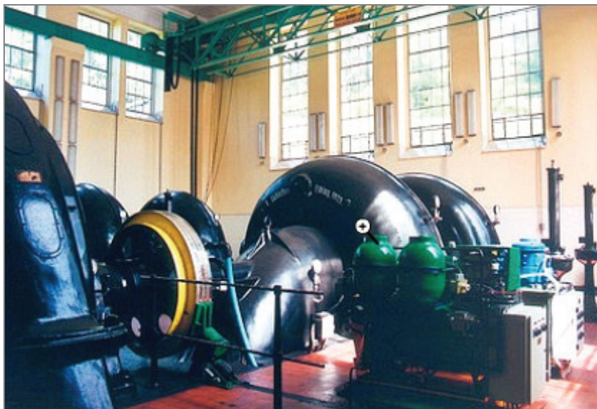
Fig. 1. View of water turbine generators in Łapino. Source: http://energia-hydro.pl/2,26,0,Galeria-Lapino.html
