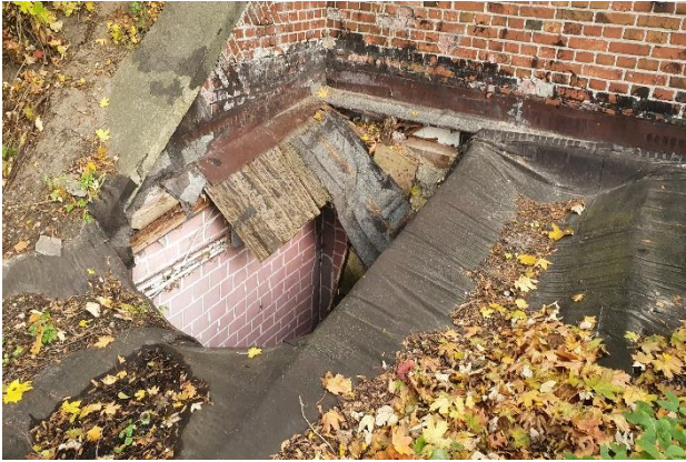
Photo. 7: Collapsed roof over former office spaces (A)
