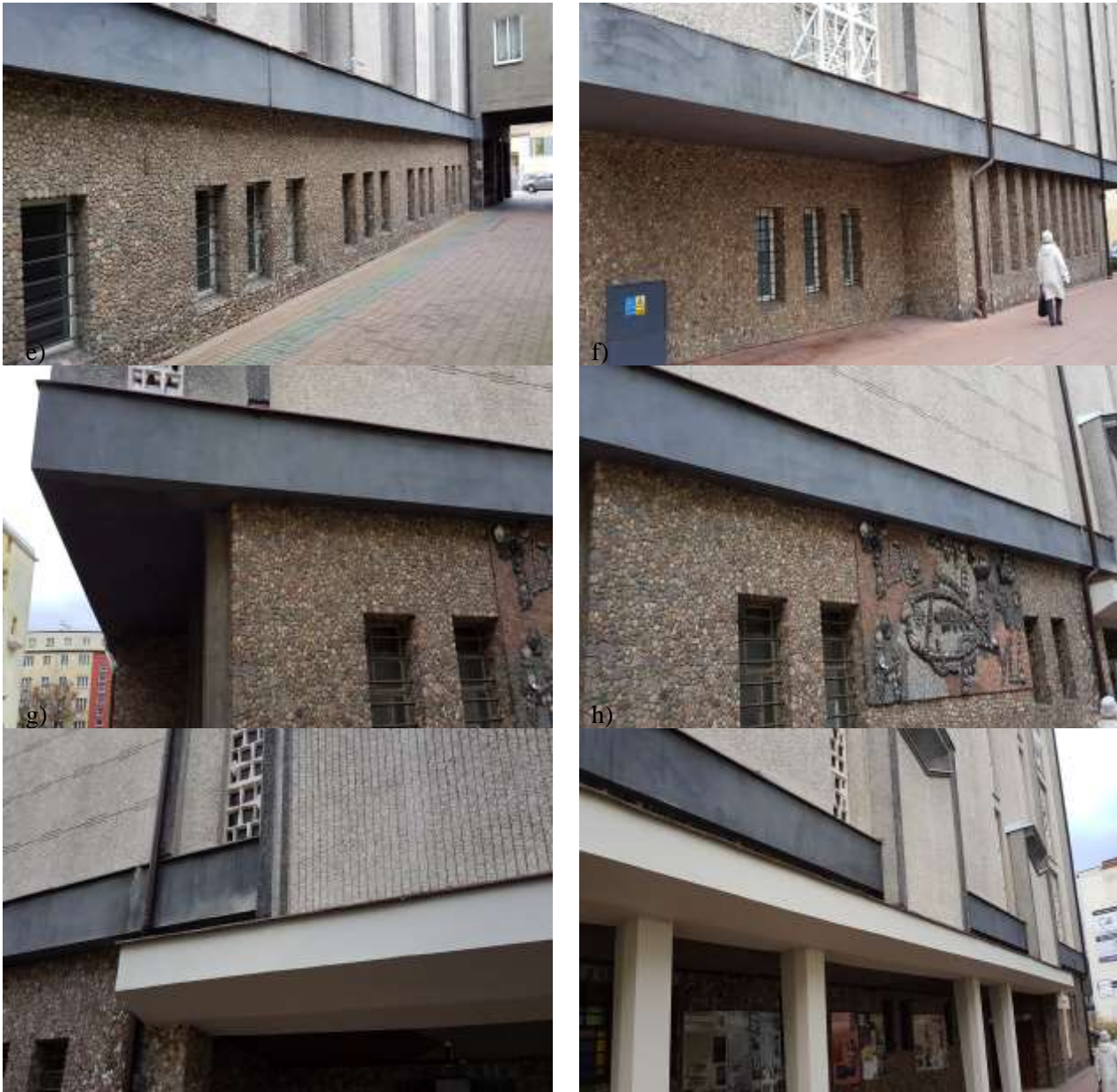
Photo 15. Base cornice after completion of renovation works: a), b) along the western elevation (from the side of 3 Maja Street), c) from the southern elevation (along Armii Krajowej Street), d) along the eastern elevation (from the side of Monsignore Hilarego Jastaka Street), e), f) from the northern elevation (along Stefana Batorego Street) (street names as of 2023) (photo by Maciej Niedostatkiwicz)
