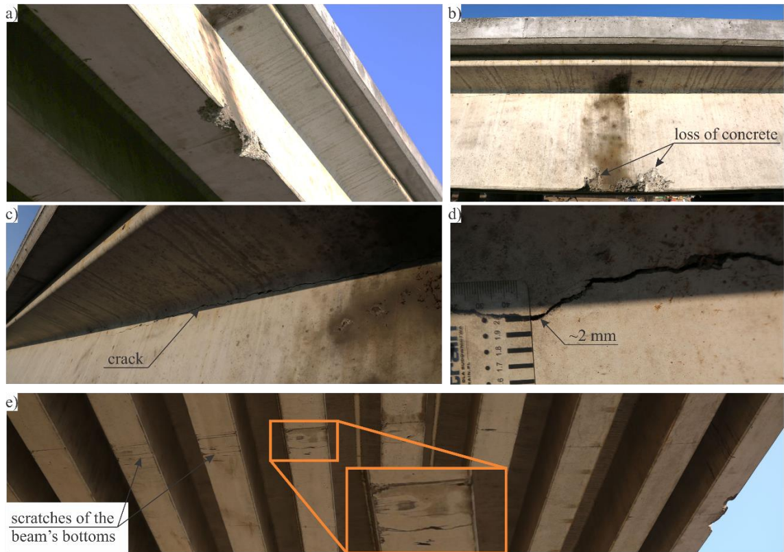
Fig. 5 The damage to the viaduct, a, b) loss of concrete (first impact), c, d) crack under flange (first impact), e) web scratches (second impact).
