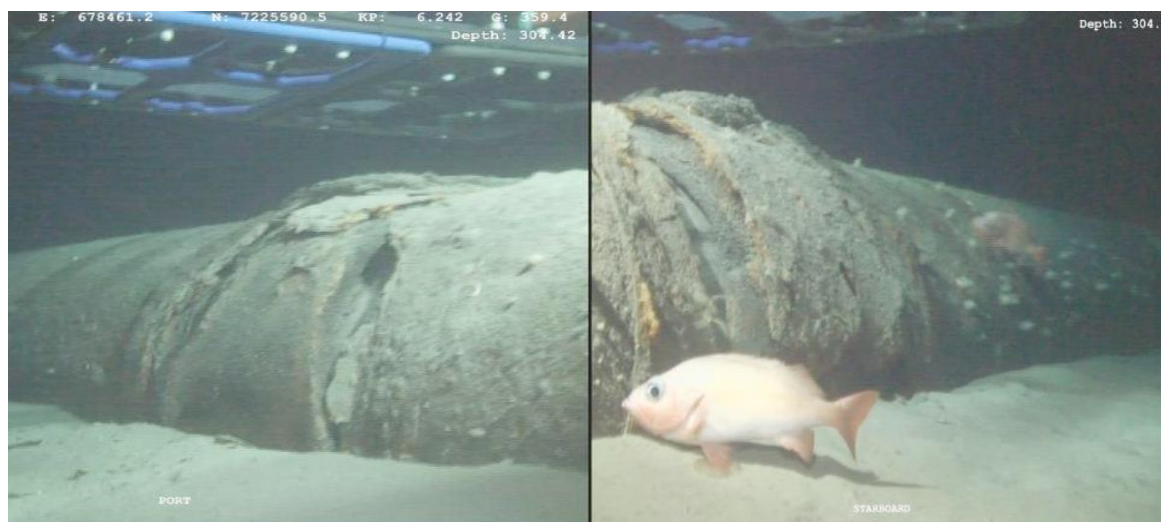
Fig. 3. Submerged pipeline observed from a ROV camcorder [11]
