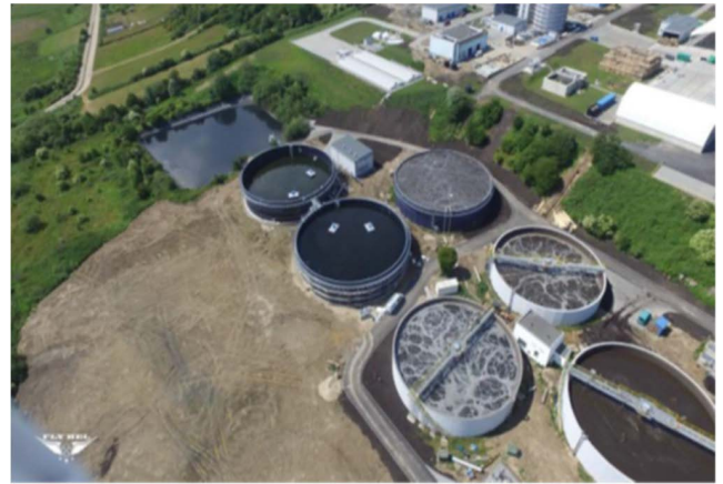
FIGURE 6. Biological part of the WWTP in Swarzewo [64].
