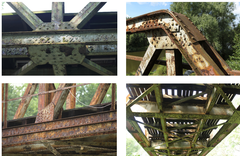
Figure 5. Bridge technical inspection – view on chosen defected elements of the railway truss bridge
