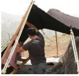
Fig. 79: Pulling up the end and the middle column which carries a ridge beam, photo.
