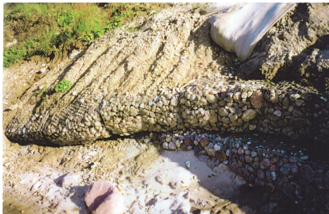
Fig. 3. Gabions composing the seawall in the region of "Bałtyk", damaged in 1998 (photo courtesy of W. Subotowicz)
