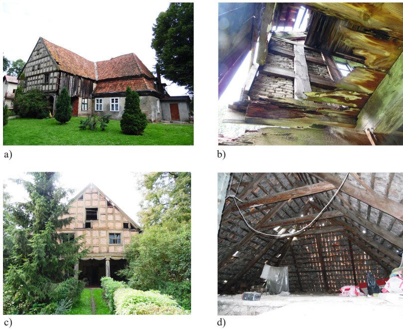
Fig. 6. Houses in: a) Steblewo 22/24, b) Steblewo 22/24 the catastrophic condition of the gable wall of the portico, c) Steblewo 15/17, d) Steblewo 15/17 leaking roofing ( photo by the author )
