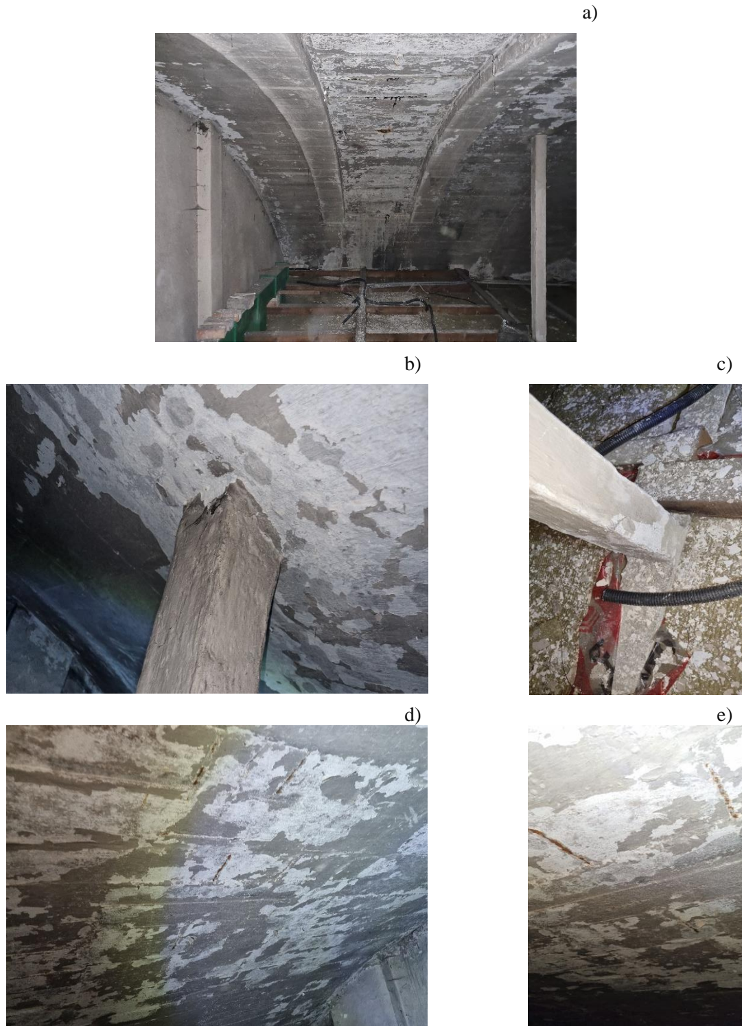
Photo 6. Warehouse building - attic space: a) stiffening ribs below the curvilinear covering slab, connection: b) post - curvilinear covering slab, c) post - horizontal tie, d), e) damage to the concrete cover of the reinforcing bars of the curvilinear covering slab
