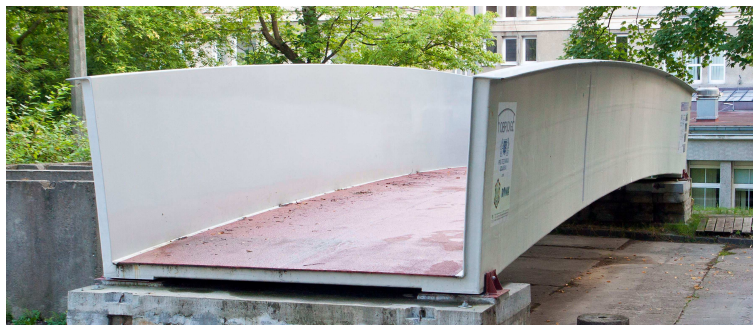
FIG. 1. Overall view of the footbridge located at the Gdańsk University of Technology campus.
